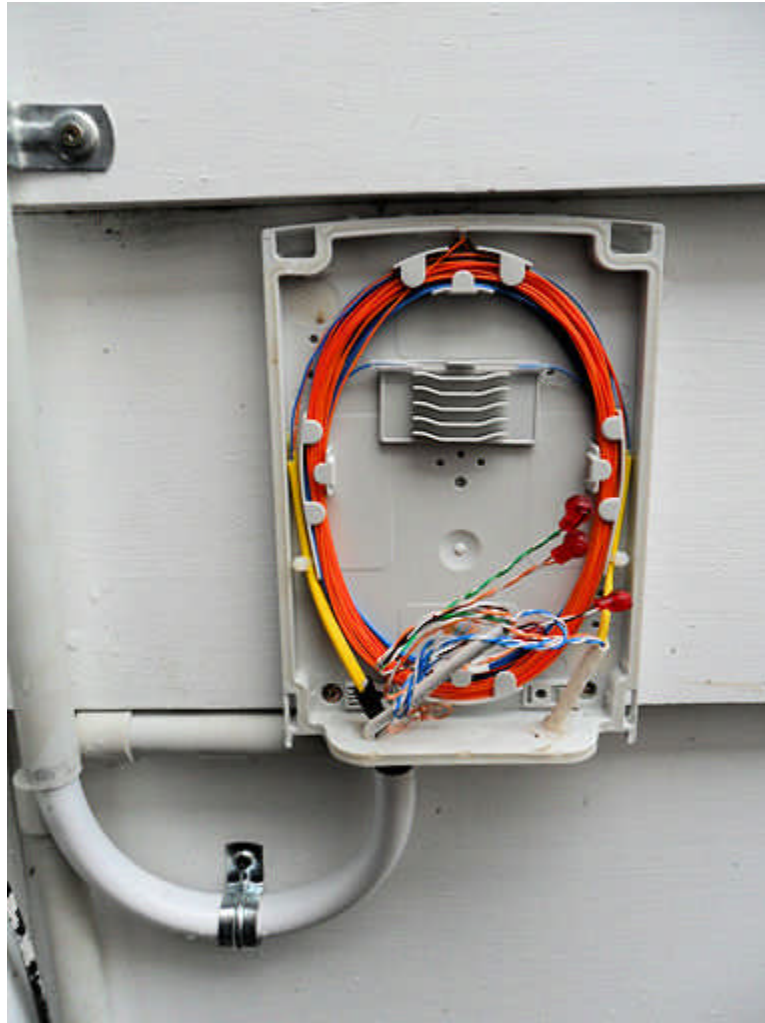
Photo 3: External Termination Point (ETP) on outside wall of house
